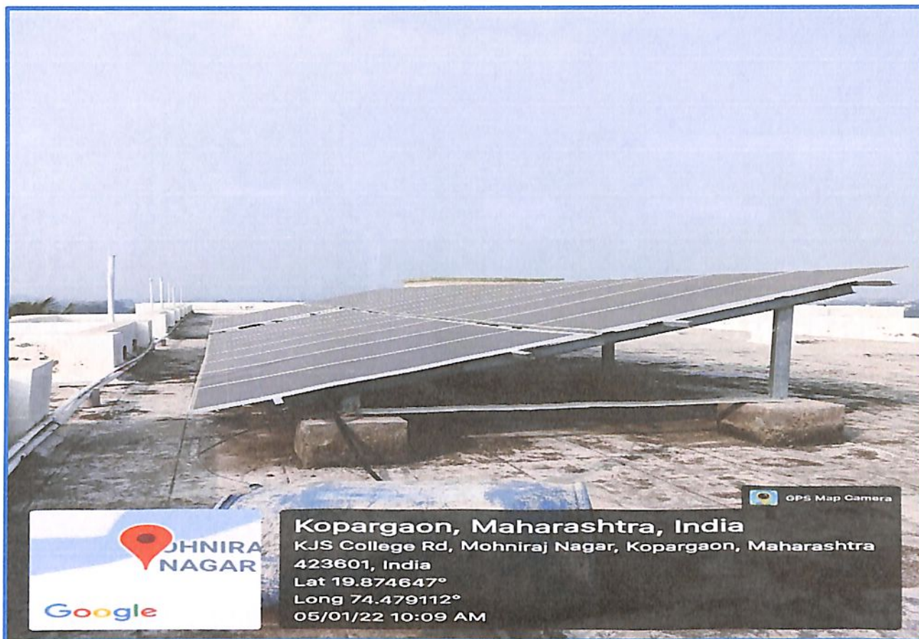
10KW Solar PV System Installed on Roof Top of Science and Technology Building
