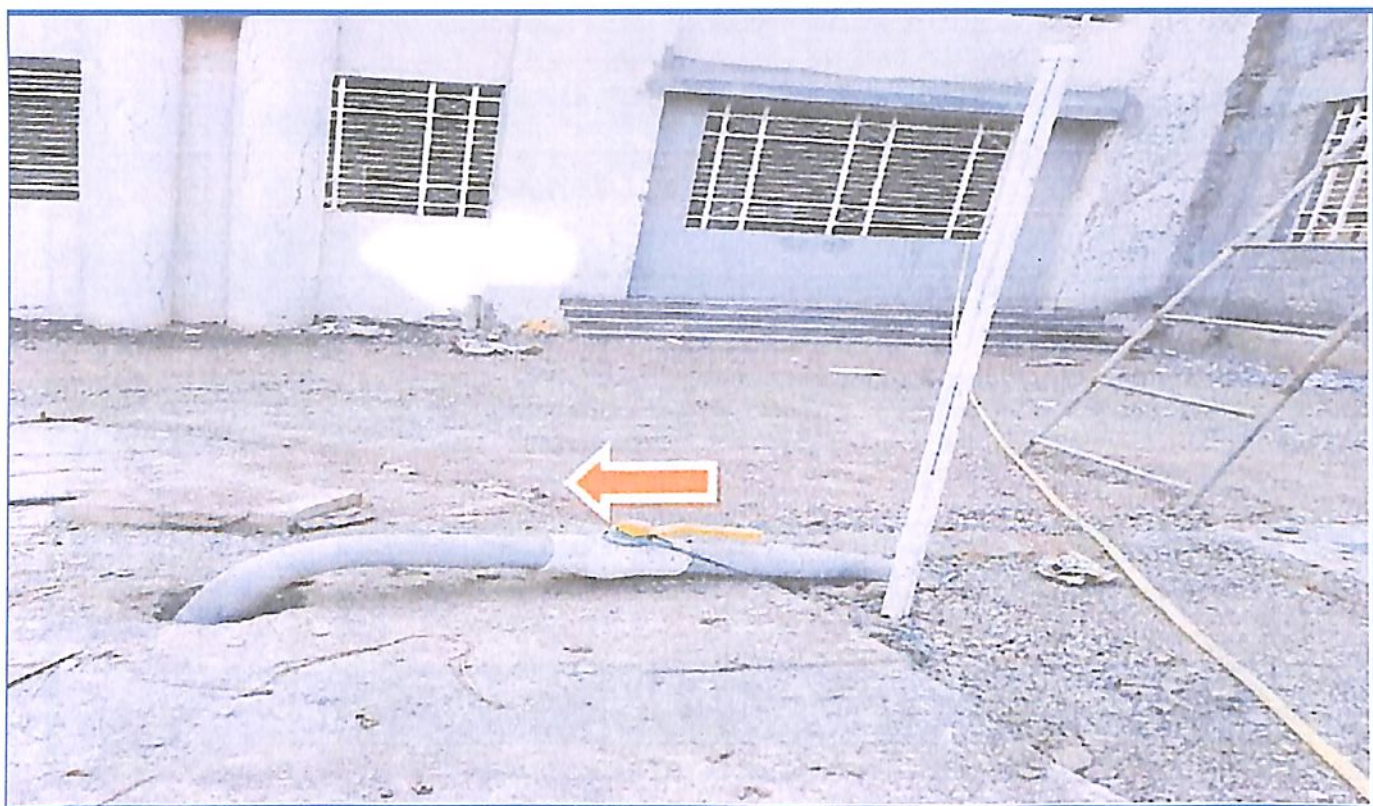
Rain Water Harvesting Structure (Inlet Pipe) at Science Building
