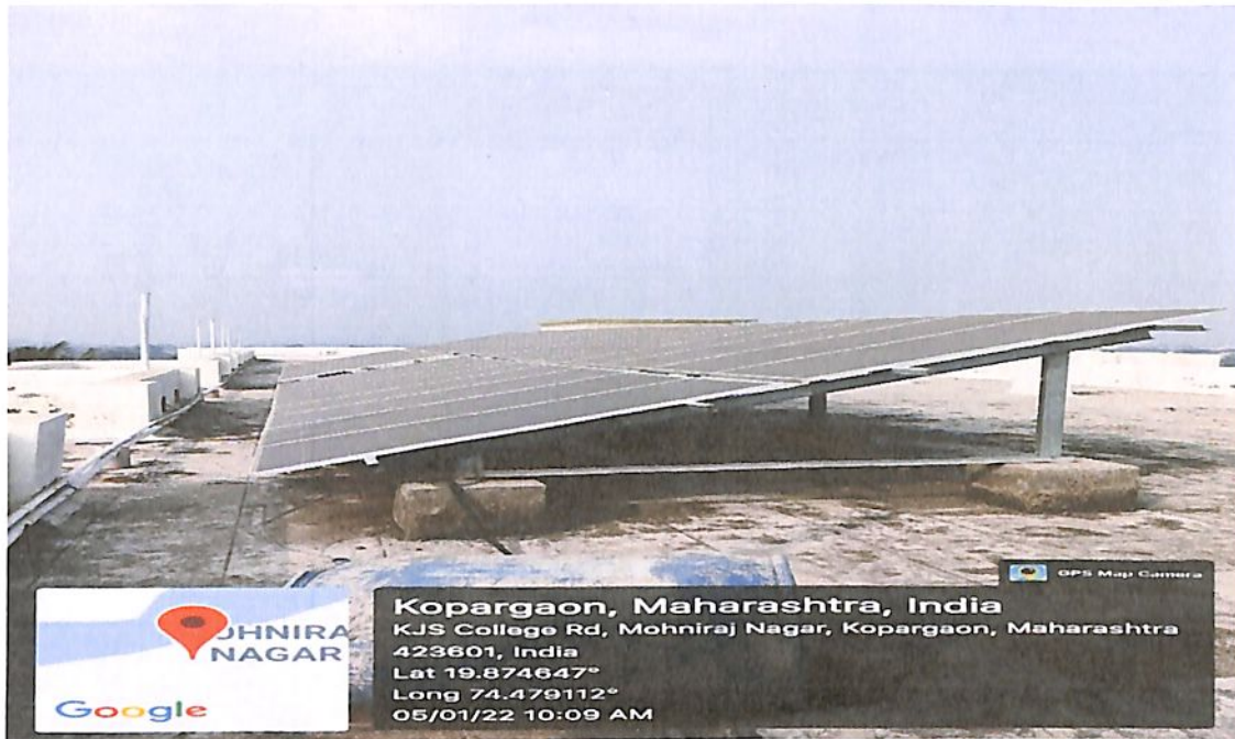
10KW Solar PV system installed on roof top of Science and Technology building.
